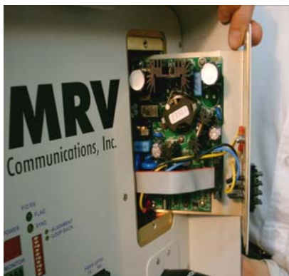
Figure I.2: Pulled out Power Supply
